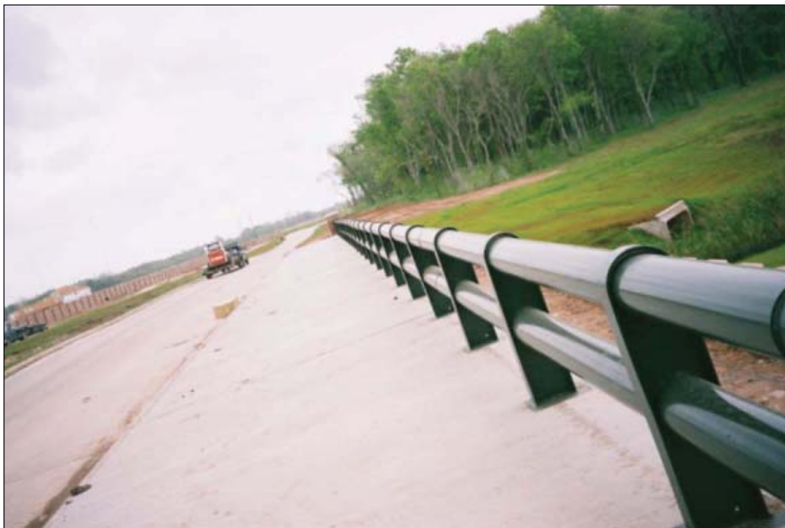
This 8-in. OD steel pipe used as bridge guards was reclaimed from a recovered pipeline installed in 1923 (Fig. 5).
