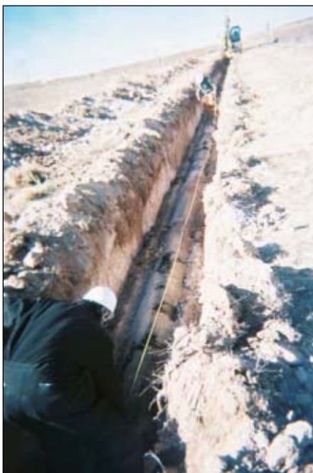
Proper recycling requires proper removal and careful measurement of the pipe. These men are measuring from weld to weld to ensure correct cuts (Fig. 2).
